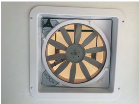
High Output Attic Fan in Bathroom
